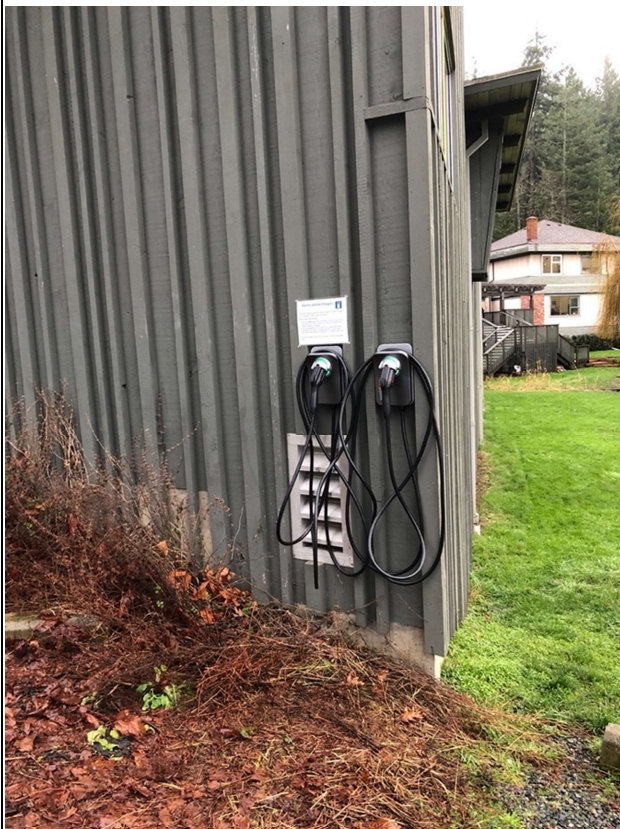
2 Level 2 EV chargers
